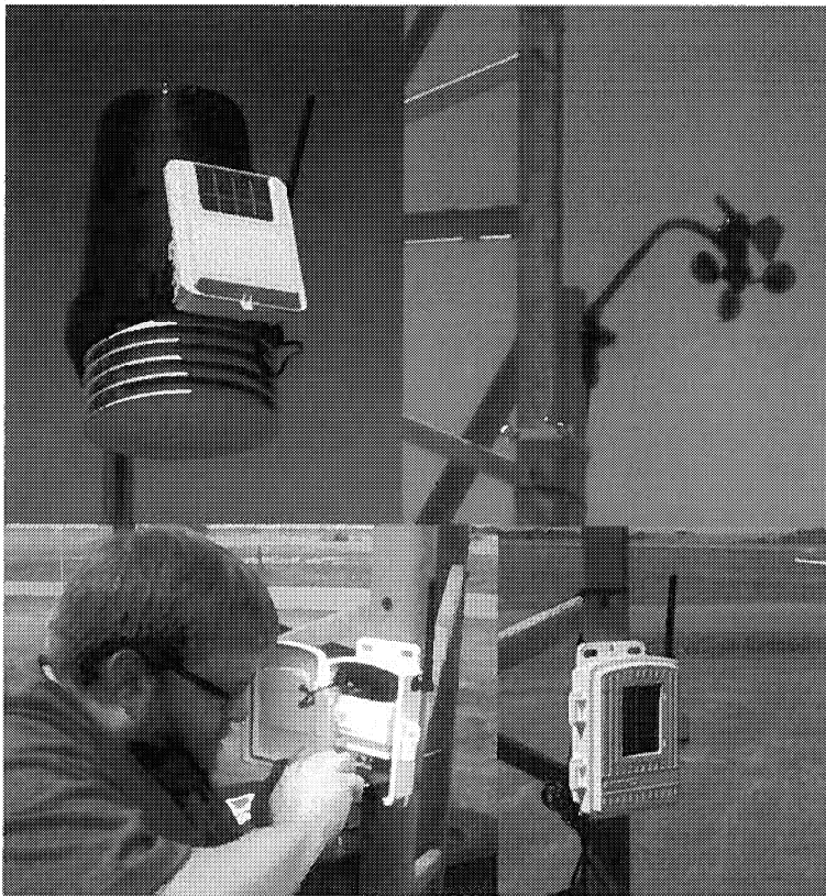
Fig. 22. The new Davis weather station deployed at the Operations Centre in 2013 is shown. Components are: Precipitation gauge, temperature, and humidity sensors (upper left), wind vane and anemometer (upper right), and wireless transmitter from wind tower to the operations room (both lower images). Wireless transmitters at both sensors allow the instruments to be placed at optimum locations, rather than compromises often made to afford wired connections directly to the office.
